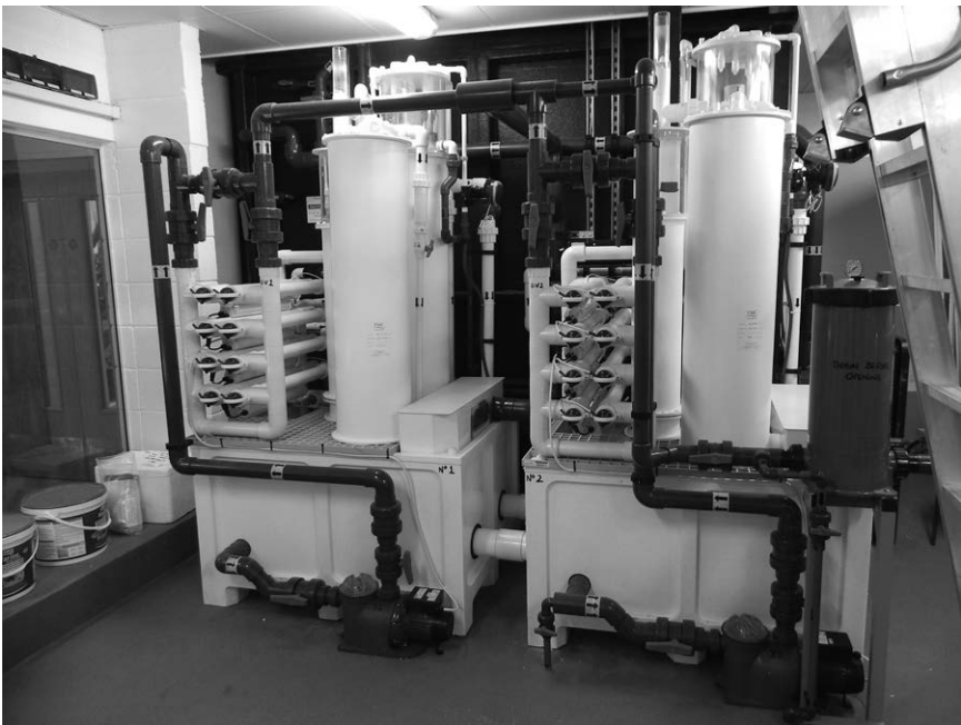
Fig. L2 Life support system for a marine tank.
