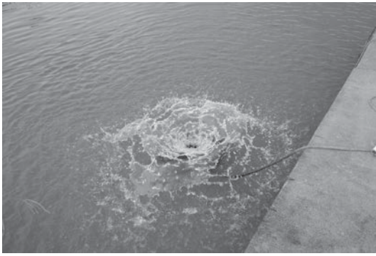
Fig. 4.5. A fountain aerator.
