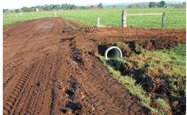
Figure 8-7 The elevated track should have drainage ditches on either side. (Courtesy of J Malmo)
