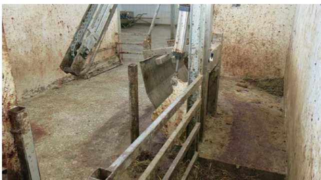
Fig. 12.19. Infrastructure left to decay. (Image credit: Paul Whittington, AWT, 2017.)
