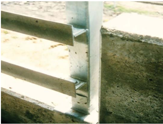
Fig. 15.5. Edges with a small diameter such as steel angle irons are more likely to cause bruises than larger rounded surfaces. Steel T shapes and angles are not recommended for lairage construction.
