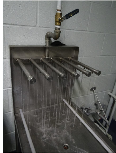
FIGURE 3.13 Devices are available to fill many water bottles at once when manual filling is needed.
